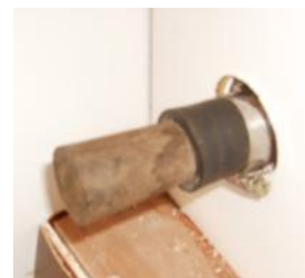
Blanked off fitting will require removal if not commissioned.
